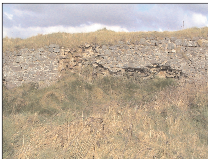
Figure 37. A general view showing length of damaged masonry along the seaward side of the main ramp. The sharp vertical left hand edge of this damaged section aligns exactly with the crest of the main ramp incline.
