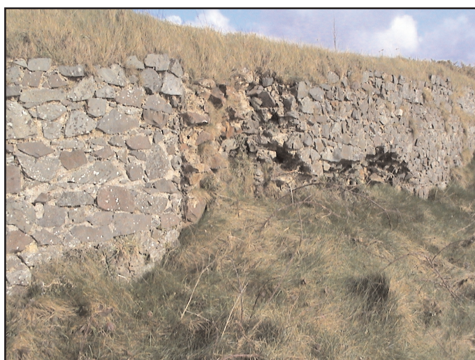
Figure 38. A close up oblique view of the damaged section shown in Fig. 37, showing the remnants of a wall tied in at right angles to the ramp.
