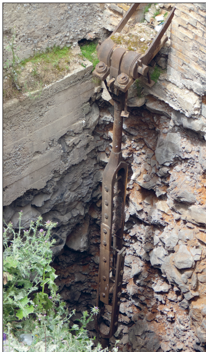
Figure 23. Pitwork attached to an angle bob leading to a balance box pit at Chalk's No. 3 Shaft near Carisbrook
