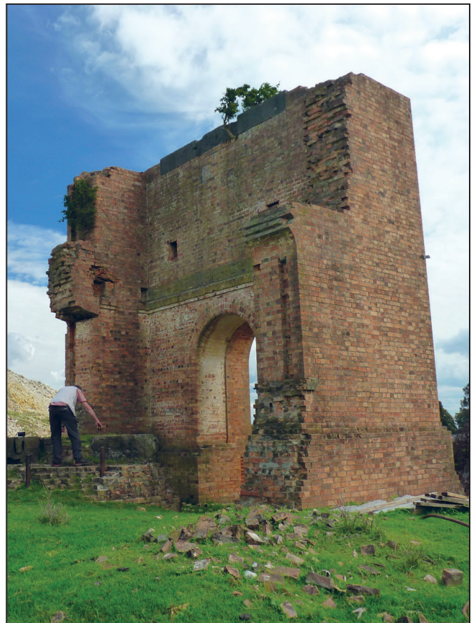
Figure 18. The huge pumping engine house on the Hepburn Estate Mine on the Berry Deep Leads near Smeaton
