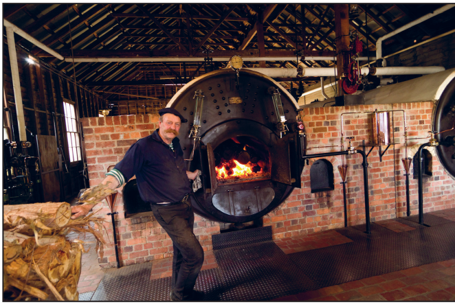
Figure 2. One of the volunteers at Sovereign Hill proudly shows off the fiery interior of a Cornish boiler
