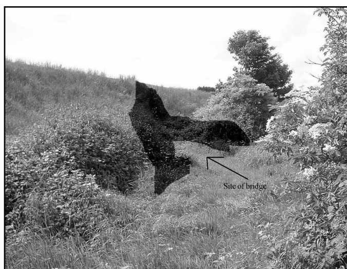
Figure 10. The location of Ballyrairie underbridge (highlighted). The arch has been filled in but stonework through the vegetation reveals its position.
