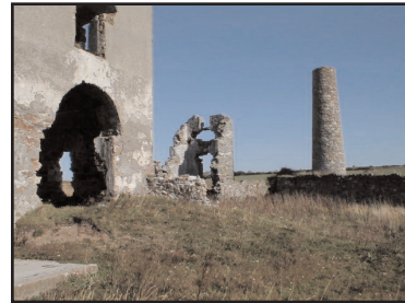
Figure 9. Damage was done to the front door in pulling out the cylinder and beam which were sold for scrap. Only the conserved shells of Tankardstown engine houses now remain.
